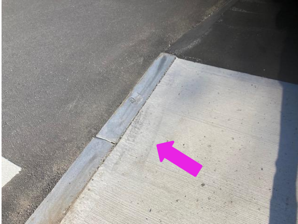
The cement sidewalk at the Westwood/Fox Hill Road crosswalk has tire marks.
