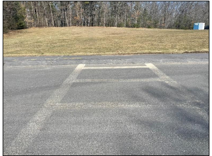
Photo 16: There is not an accessible ramp at the north side of the crosswalk at Fox Hill Road and Westwood Street.
