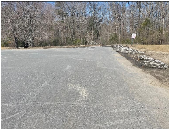
Photo 17: Striping within the parking lot directing parent traffic is faded.
