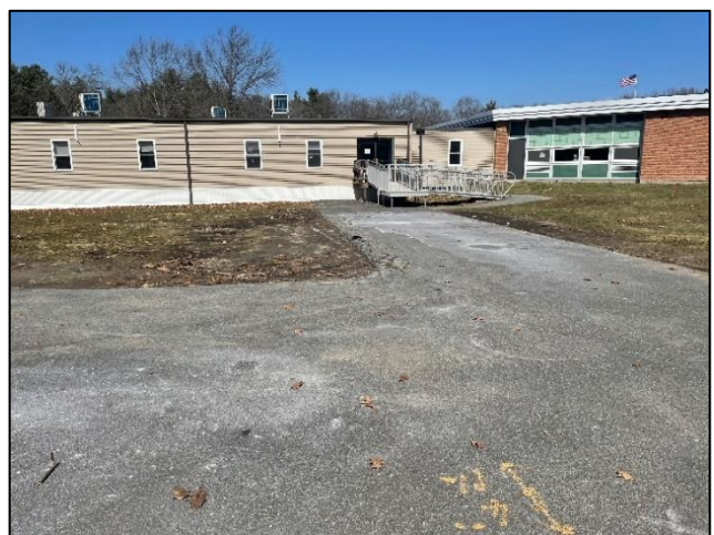
Photo 10: One school van was observed unloading at the rear of the building at the accessible ramp.
